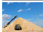
"Wet Sand Pile" is a simple but critical innovation for completions efficiency & Trimulfrac
